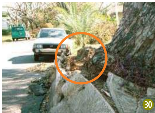
Figure 30 This leaning tree needs to be removed since major structural roots were broken and lifted.
