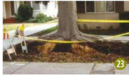
Figure 23 Construction is especially damaging to roots, such as these roots cut during curb repair.
