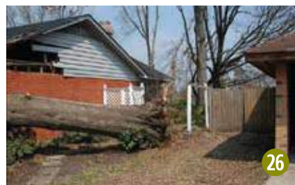
Figure 26 These white oak roots were confined by the buildings around them, probably damaged by construction and compaction, resulting in a root system too small to support such a large tree canopy.
